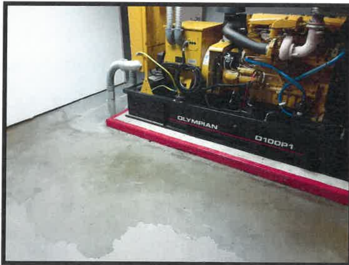
Flooded LEDU Basement shop vacuumed during each rainstorm. Water flows directly towards an emergency generator.
